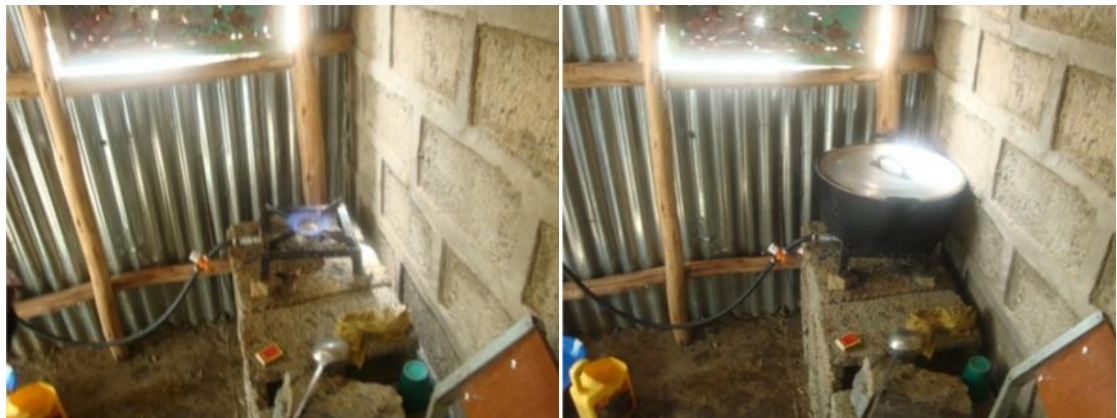
Cooking Stove by Biogas Digester installation in Mekele Elala Nunnery
